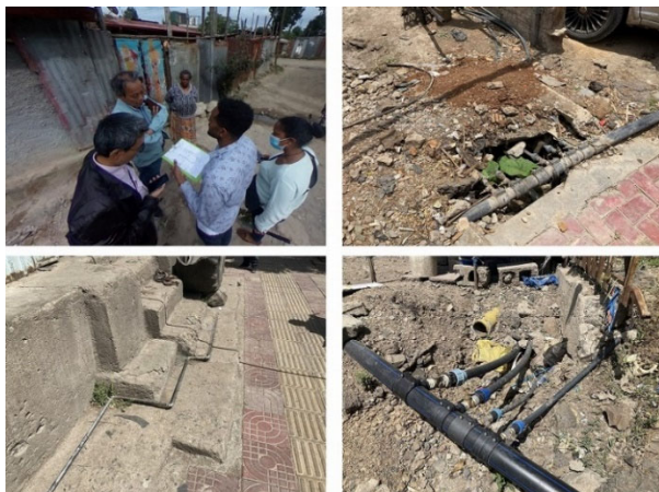
Photo 1 Situation of exposed piping and spaghetti pipes
