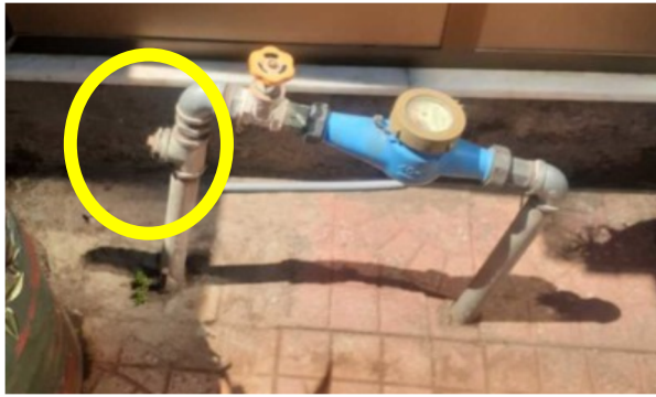
Photo 6 Example of a branch installed upstream of a water meter
