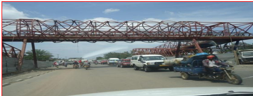
Pedestrian crossing and widening of two lanes to three lanes road in 2013 by Regional TANROADS (Mabatini)
