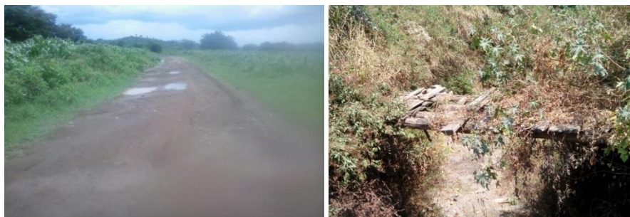
Part of impassable road in Maendeleo ward and the Nkunywa bridge before construction
