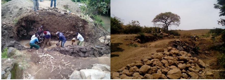
Community excavating the Nkunywa bridge foundation and Rock excavation in road upgrading
