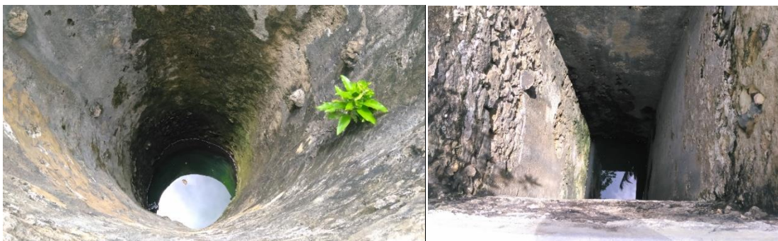
Unsafe water wells in Chole Village
