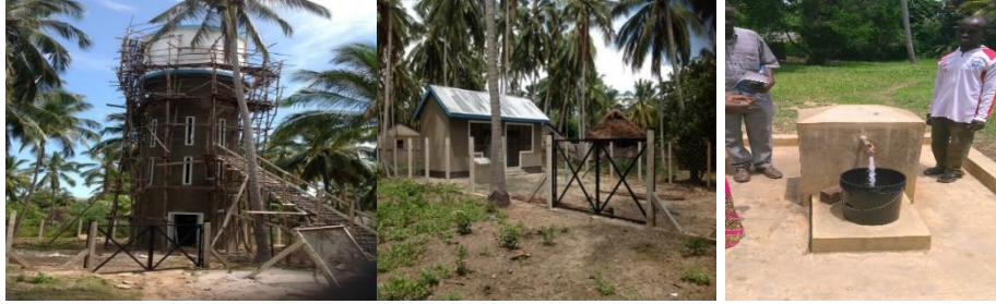
Water tank, pump house and distribution point
