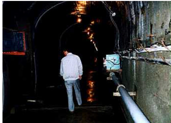
The inspection tunnel which passes through the dam (the tunnel is equipped with devices to detect distortion of the dam, water loss and other problems)
