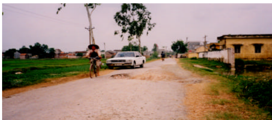
Photo 1 The road has been damaged by large trucks working on dyke construction
