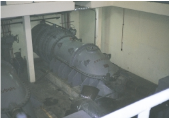
Large-sized Pump installed by this Project
