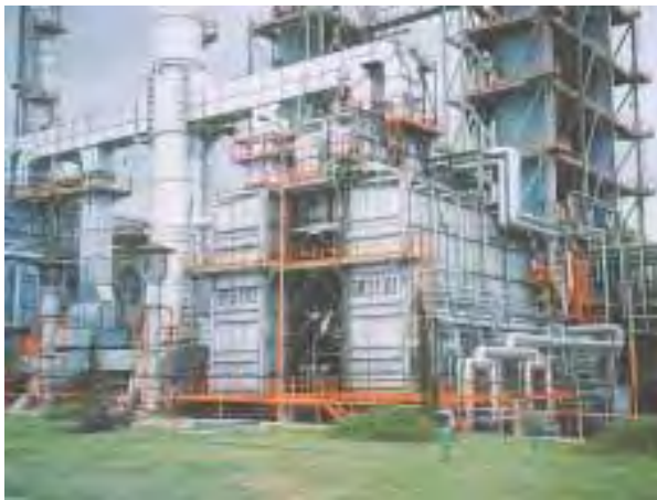
Introduction Facilities : HDR Equipment in Tula Oil Refinery
