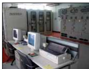
Fig.3. Control Room in Substation
