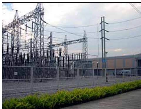
Mae Lao Substation constructed under the project
