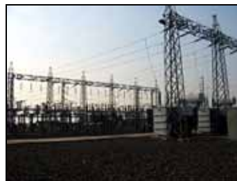
Fig.2. Laeme Chabang Substation
