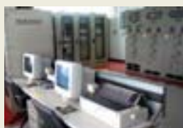
Control room in substation
