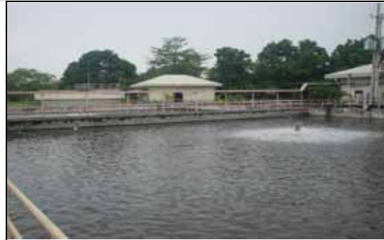
Project-installed sewage treatment facilities
