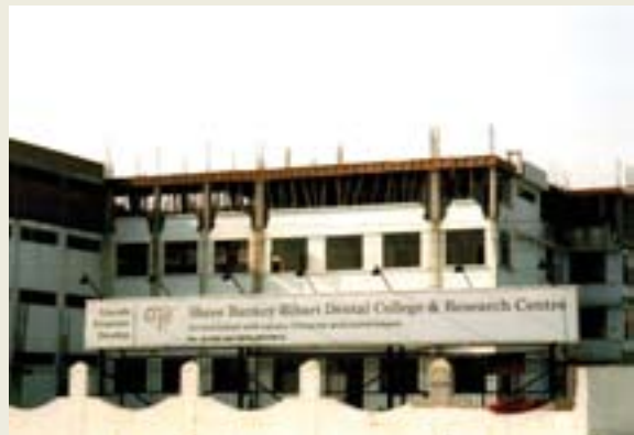
Dental college under construction near the road following the completion of this project
