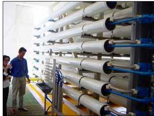
Jerba Desalinization Plant
