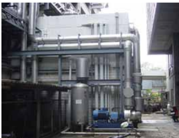
Heat condenser equipment installed at EGAT
