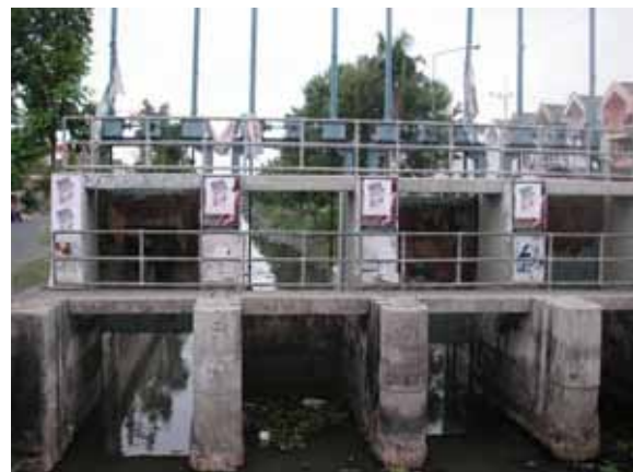
Water Gate of Improved Kubong Agung Canal
