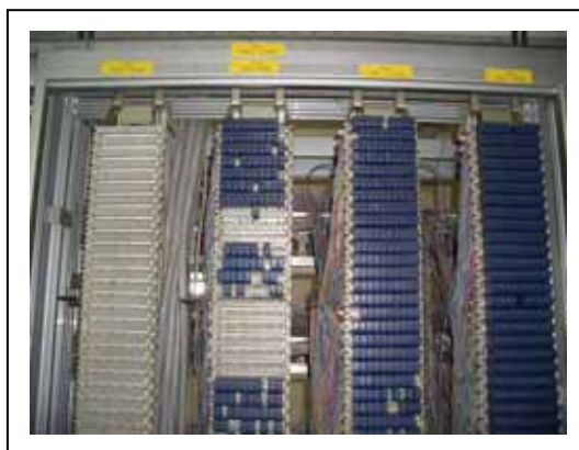
Switchboard installed under the project
