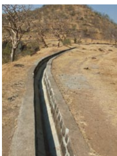
Drainage system above the Ajanta caves
