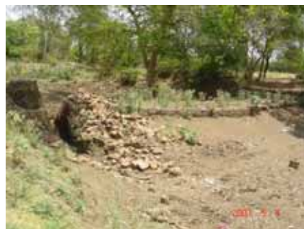
Figure 9: A damaged CAT structure
