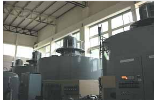
Figure 1: Umiam Hydro Power Station Stage I
