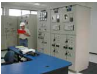
Figure 8: Daily Management inside a Transformer Station
