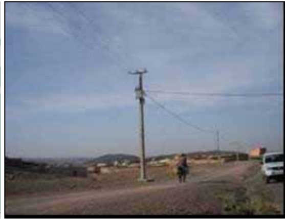
Improved electricity grid
