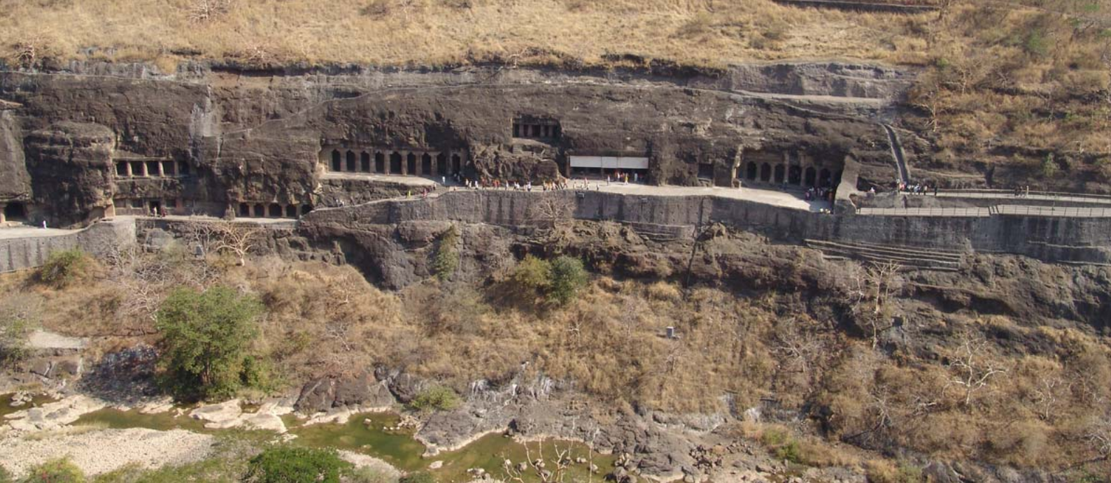
(Figure 10) High concrete-made retaining wall which has appeared as a result of the pathway expansion
