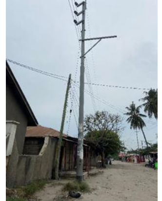
33kV Distribution line
