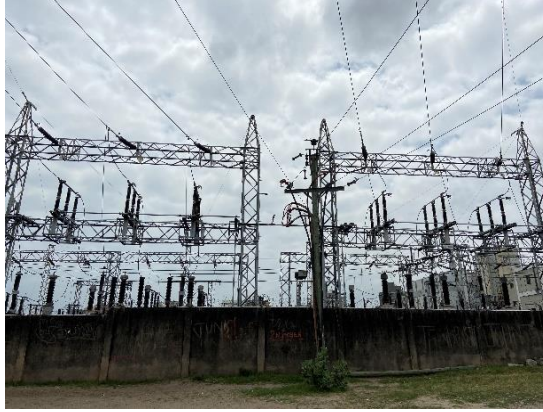
132kV Transmission line gantry (Ilala substation)
