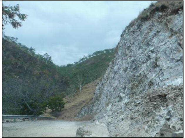
Photograph 4 Dili to Manatuto – Km 44.0 Landslide
