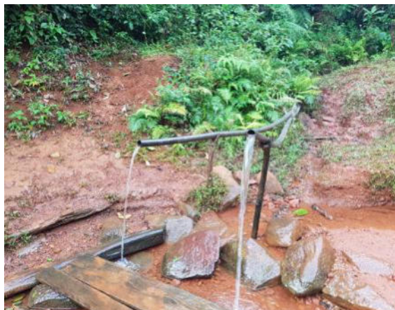
Gravity-fed water system in Xiengluang Village
