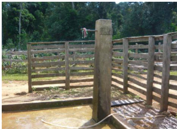
Gravity-fed water system in Prao Village
