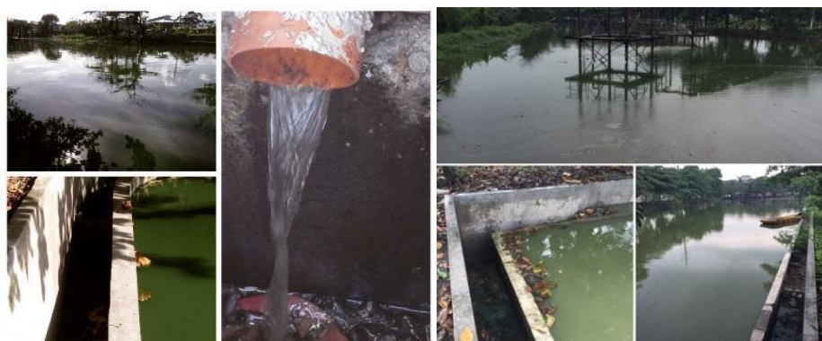
Photo: Lagoon and discharge from the pilot septage treatment plant (Left: March 2015, Right: Septemeber 2015)
