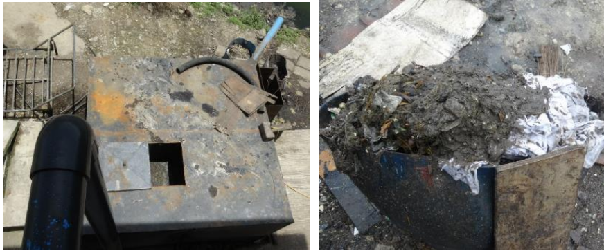
Photo: Septage receiving tank temporarily placed to remove solids in septage and removed solids
