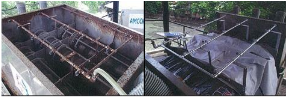
Photo: Dewatering press become rusty and after providing protection (Aug, 2014)
