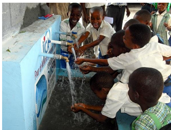
Fig. 8: A public water tap installed by urgent rehabilitation works after the major earthquake in Haiti
