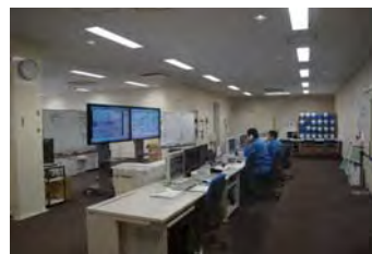
Kawai Purification Plant by PFI Scheme, (BTO) Yokohama City
