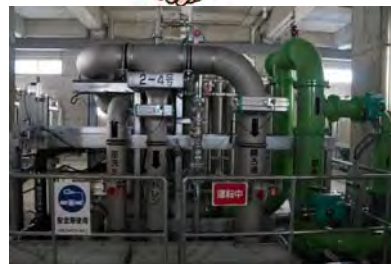
Inside of water purification plant "CERAROKKA"; built by PFI scheme in Yokohama
