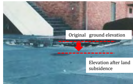
Depression caused by land subsidence https://www.pref.saitama.lg.jp/a0505/901-20091202-17.html
