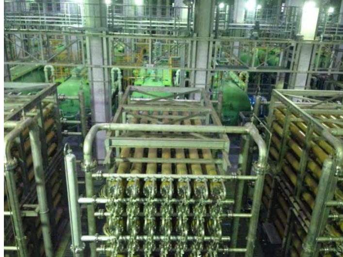
Photo 3. Seawater Desalination Facility in Chatan Water Treatment Plant (February 25, 2016)
