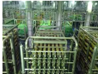
Seawater Desalination Facility in Chatan Water Treatment Plant
