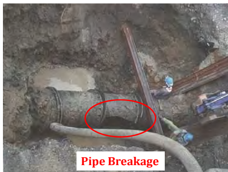
Source: JWWA, "Casebook of Water Supply Accidents for Practical Use," 2008. Note: Photo is modified from original (indicated in red)
