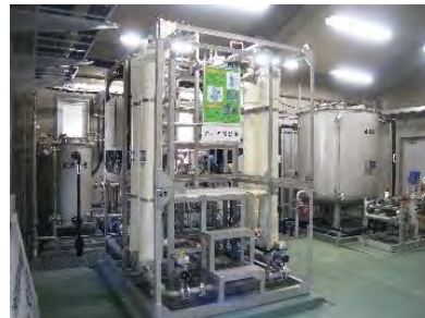
Membrane filtration facilities, Water supply system for Kuroda area in Kyoto city, Waterworks Bureau, City of Kyoto http://www.city.kyoto.lg.jp/suido/page/0000160981.html
