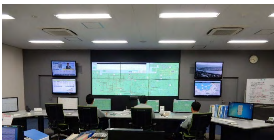
Photo 3. Fukuoka City Water Management Center, taken on April 19, 2016
