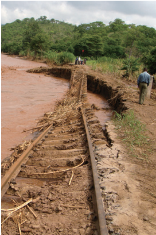
The railway track are planned to be relocated to the area where an erosion can hardly reach.
