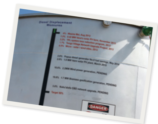
Diesel fuel tank at the Popua power plant. Electricity is delivered everywhere on the island from here.
