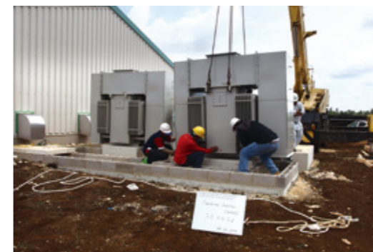
Workers install transformer panels, which function as electric transformers to supply power to all regions.
