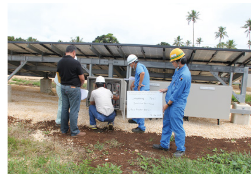
Sato checking wiring of solar panels with local workers for the test-run.
