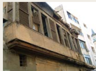
Aging building in Qanawat
