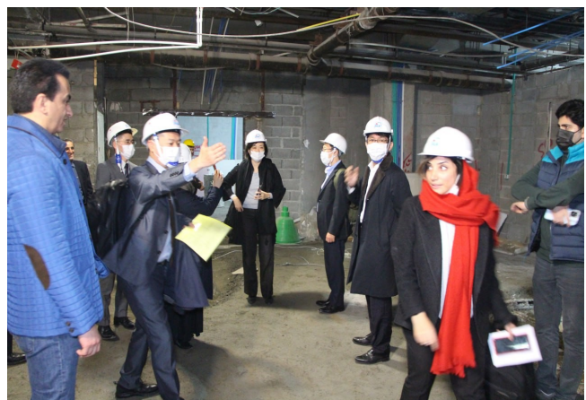
• Visiting the progress of construction and installation of medical equipment in Arash Women Hospital
