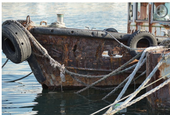
Rust on the surface of a ship
