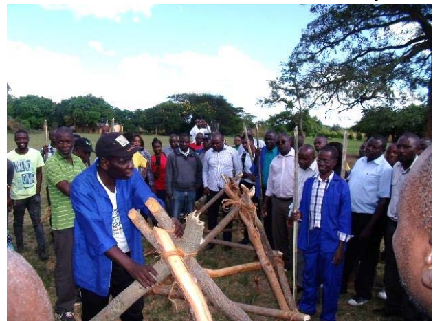
Demonstration of simple weir construction instructed by the masters of trainer team (left person). After this demonstration, the participants practically constructed the weir on the river nearby (KOT in Copperbelt Province)
