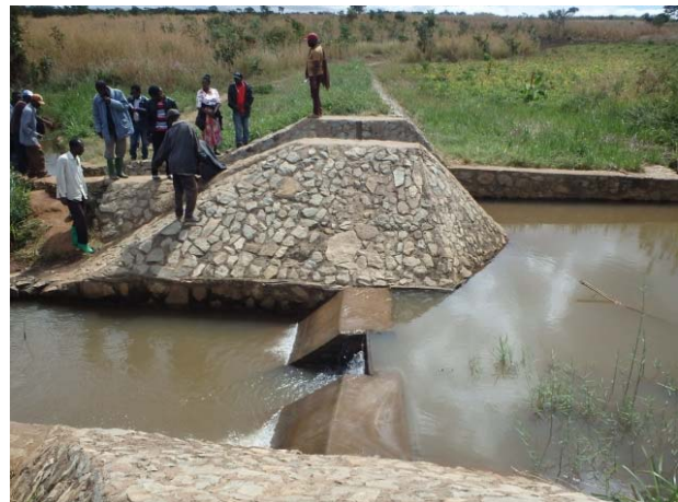
Most of the permanent weir sites are well-maintained (Musanza scheme, Nakonde District, Muchinga Province)
