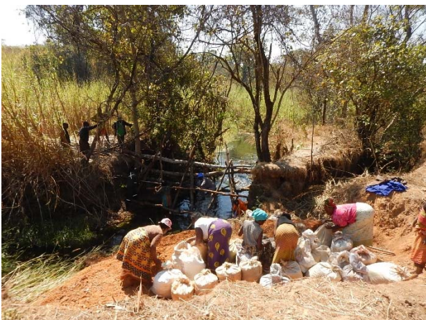
While the male farmers fabricate the frame of trigonal weir, female farmers prepare sandbags which are put in front of the weir. London Irrigation Scheme in Chilambe Camp, Kalulushi District, Copperbelt
