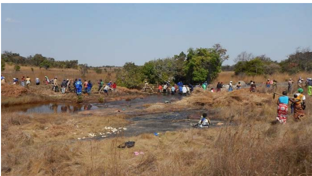
Weir construction works were shared. Male farmers fabricated the frame of trigonal weir and female farmers prepared grass and ishinde. Chiefteness Serenje Camp, Serenje District, Central Province
