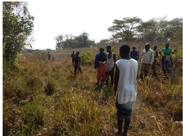
Determination of alignment of the canal using line level. Kawiko Camp, Mwinilunga District, North-Western Province
