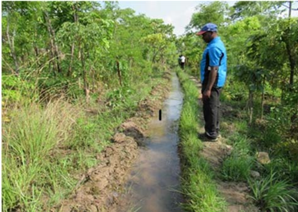
De-silting of furrow is one activity of O&M (Nsama district in Northern Province)
