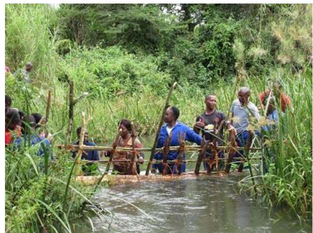
Participants practiced how to construct a simple weir, an entry point of small-scale irrigation development in the field. A picture shows construction of the inclined type. Female participants actively joined the construction as the picture shows.
