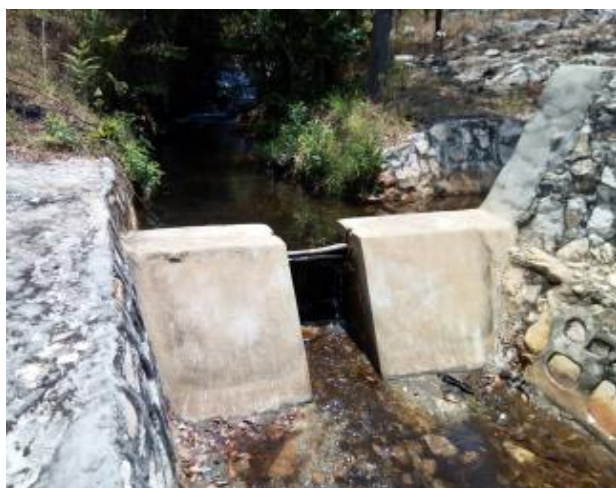
Musanda Irrigation Site in Kasama District, Northern Province, constructed by T-COBSI. Condition of the permanent weir is good, and this site is selected as E-COBSI District Model Site.
