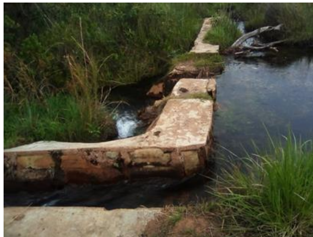
Chilala Irrigation Site in Mporokoso District, Northern Province constructed by COBSI-study. Although the weir is partially damaged, farmers can still take water from the front site furrow.
