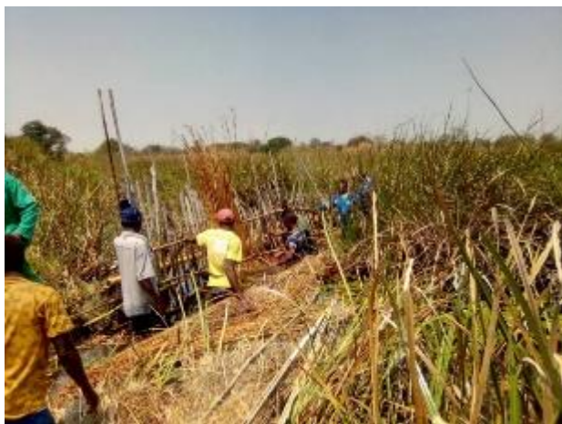
Weir construction Mambili camp, in Chingola Districts, posted by E-COBSI CBP group
