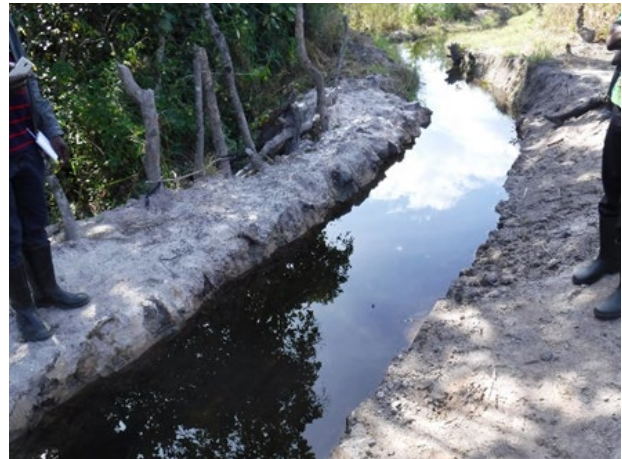
The furrow repaired by using the revenue from a demonstration plot in Kawanbwa district (Luapula province).
