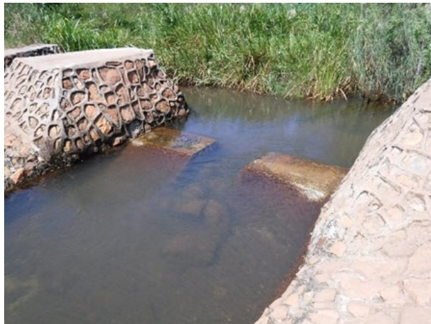
The Permanent Weir in Mpika district. Condition of the weir constructed in 2014 is still fine. (Muchinga province)
