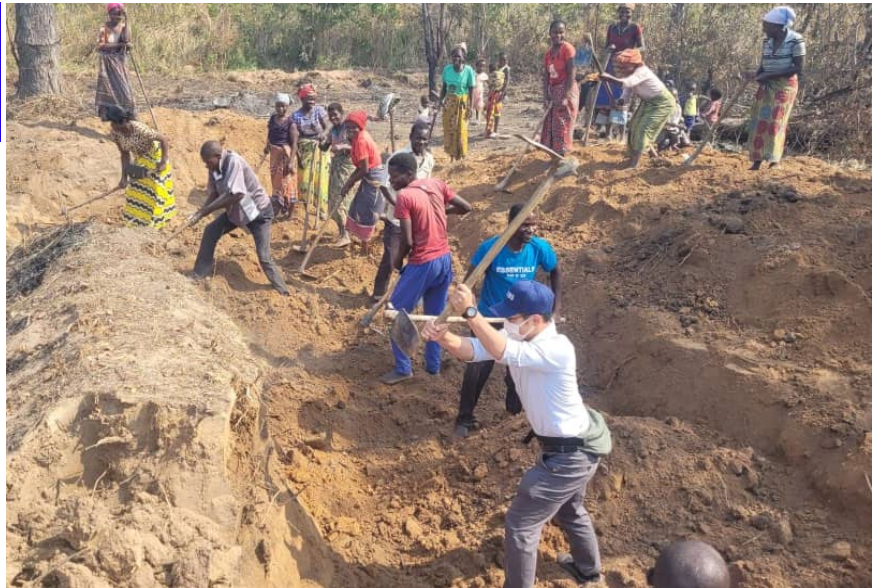
Construction of the fishpond in the district model site in Lupospshi District (Northern Province)
