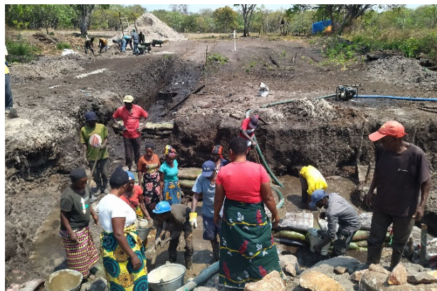
Stone masonry work in Mkusi. The project team is using a pump to drain water coming out of a ground. (Central Province).
