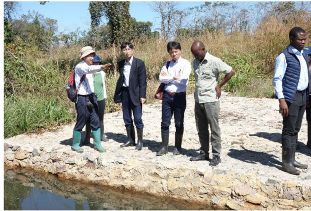
Dr. Sagawa from E-COBSI team, explained design of the permanent weir and the progress of construction. (Mufulira district, Copperbelt Province)
