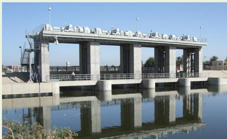
Monshat El Dahab Regulator on Bahr Yusef Canal (grant aid project for repair of the regulator completed in 2010)
