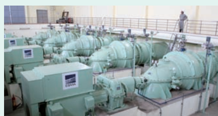
Yen So Pumping Station
