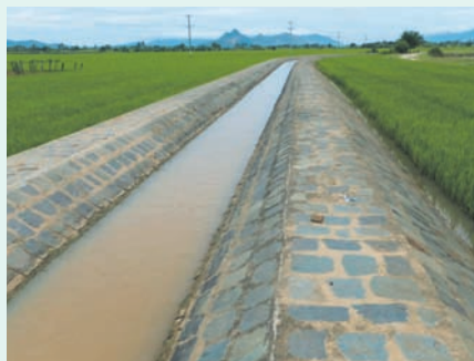
A Channel constructed by the Phan Rang Irrigation Project: The land has been enriched with irrigation water for 50 years.
