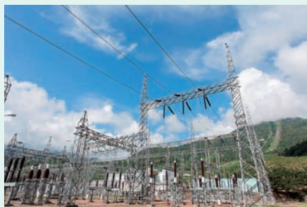
Da Nhim Hydroelectric Plant (Photo: JICA Ex-post Evaluation Report)
