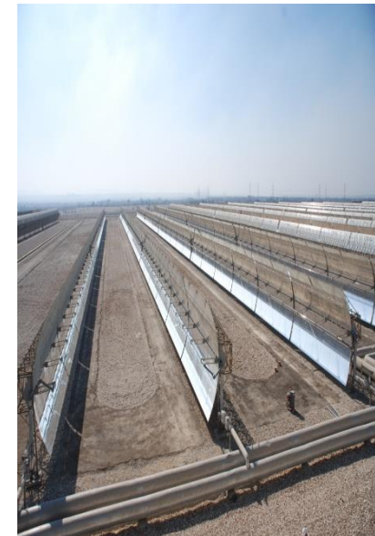
kuraymat Solar thermal power plant 20 MW (Solar Share)
