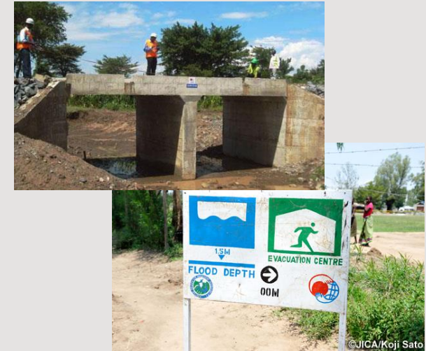
Construction of flood control facilities and training through the Community-based Flood Disaster Management to Adapt to Climate Change (Kenya)
