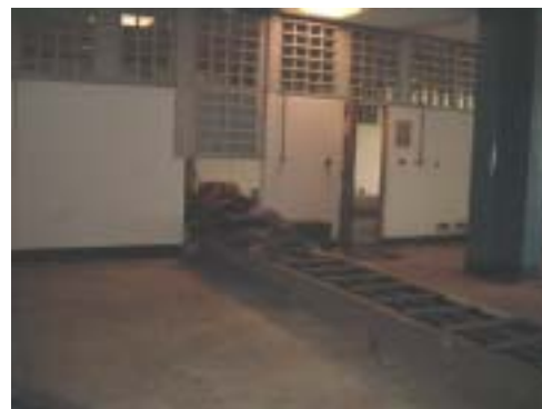
Luggage Turn 表 in Deterioration
