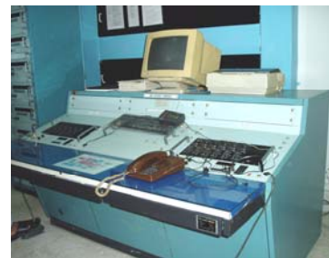
VHF Telephone Console
