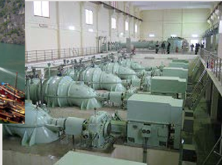
Pump station in Hanoi, Vietnam
